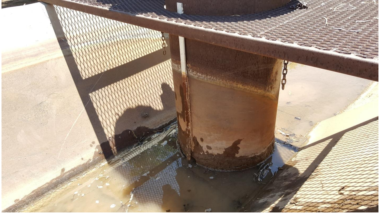
Figure 19. Close up (upstream side) of previous flume, with visible rust patterns indicating maximum water height and critical flow profile.
