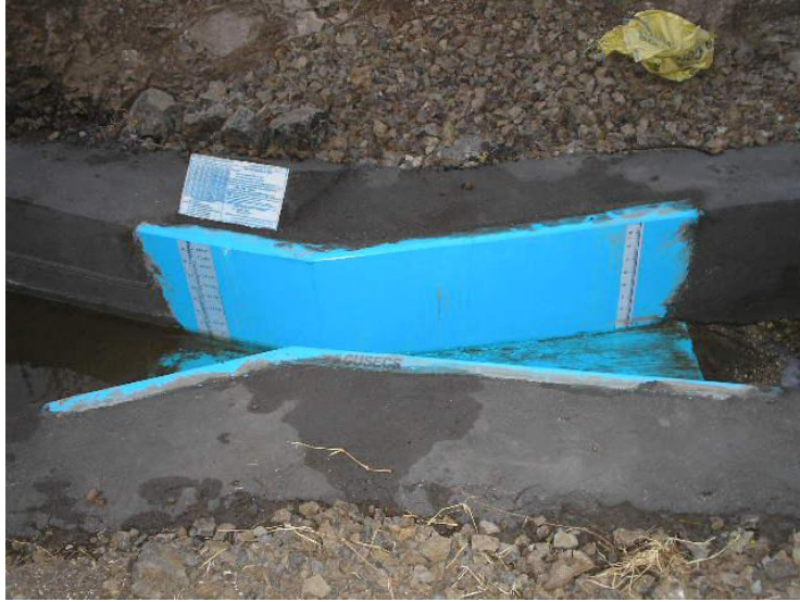
Figure 30. Installed cutthroat flume.
