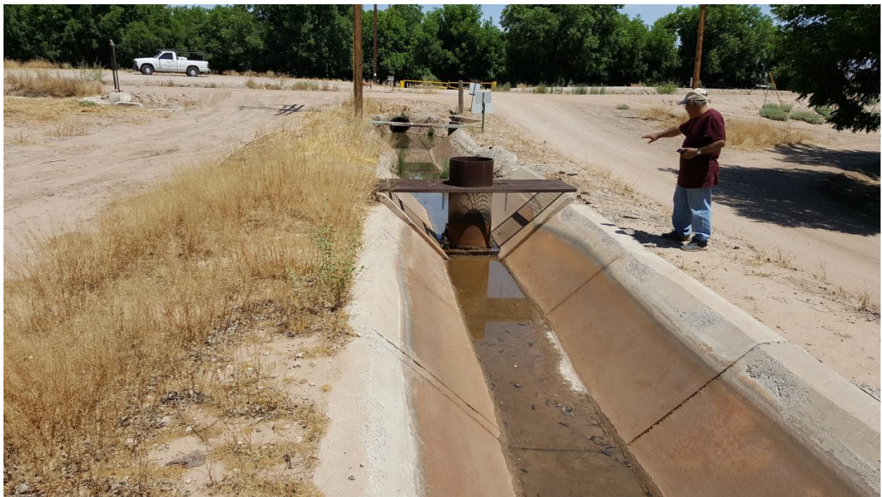
Figure 18. Trapezoidal flume in southern New Mexico Irrigation canal located at GPS coordinates: 32.391389, 106.846111.
