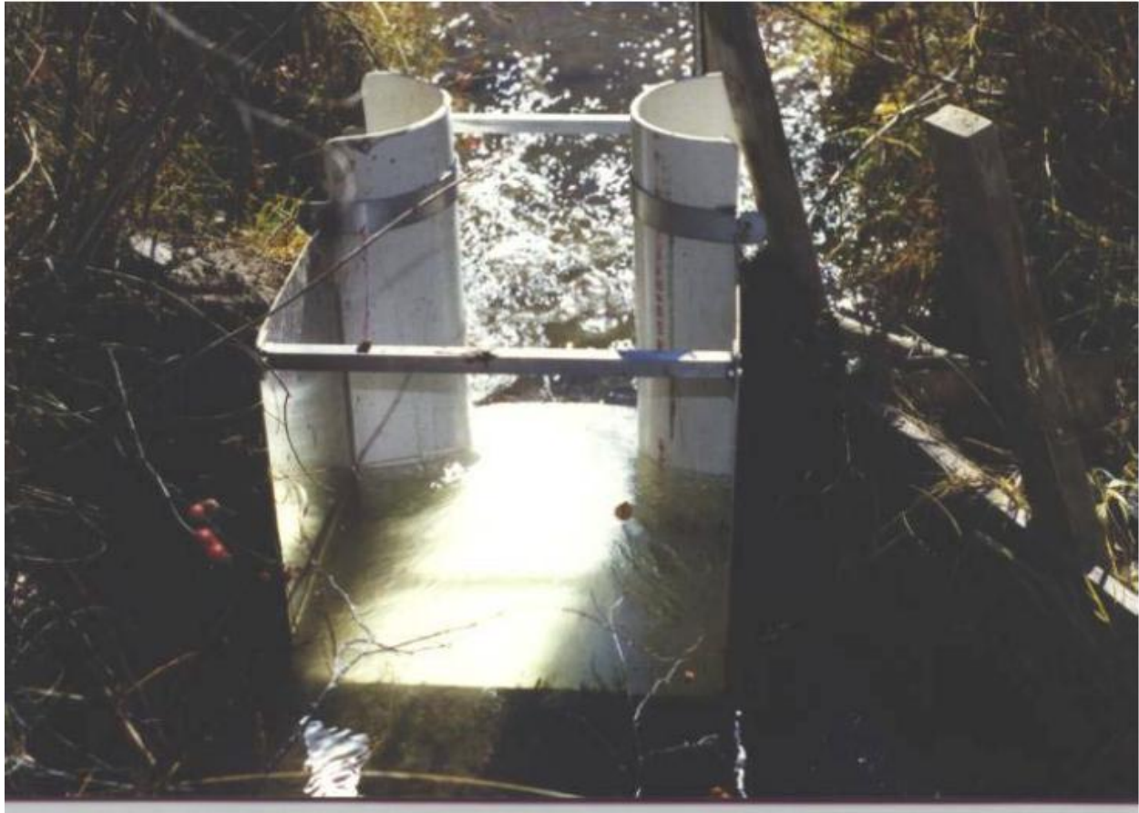
Figure 16. S-M flume installed in an acequia in Santa Fe, NM. (Samani, 2005).
