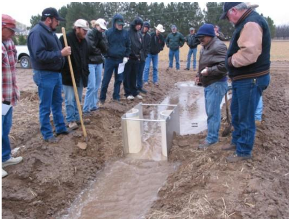
Figure 17. S-M rectangular flume installed in an unlined ditch in southern New Mexico.
