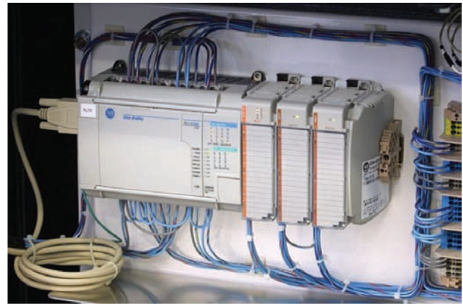
Figure 13-2 PLCs are always mounted horizontally. Source: Courtesy Rogers Machinery Company, Inc.
