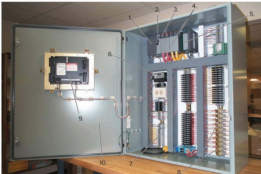
Figure 13-1 Typical PLC control panel enclosure. Source: Courtesy Aaron Associates.
